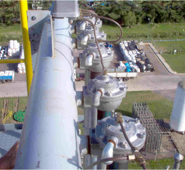
Figure 6. New header and pulse valves.
