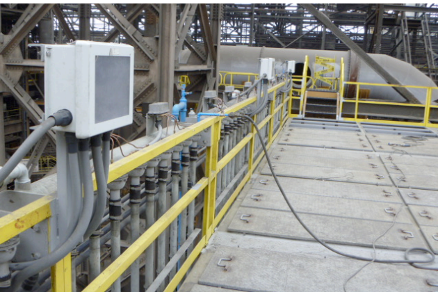
Figure 9. New controller enclosures and header and valve assemblies.
